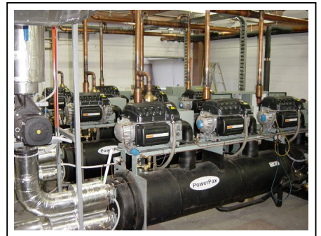
Remote air cooled chillers 800 kW
